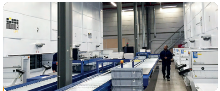
Integration with conveyors
